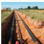
Pipelines in France. © Ineke Scholte
